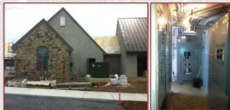
The left image shows the new transformer outside of the ground level mechanical room. The right image shows the primary distribution center in that room.
