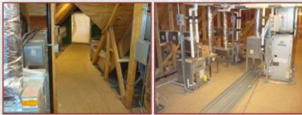
The left image is an example of the catwalk common in the mezzanine. The right image is heat pump group for a wing.
